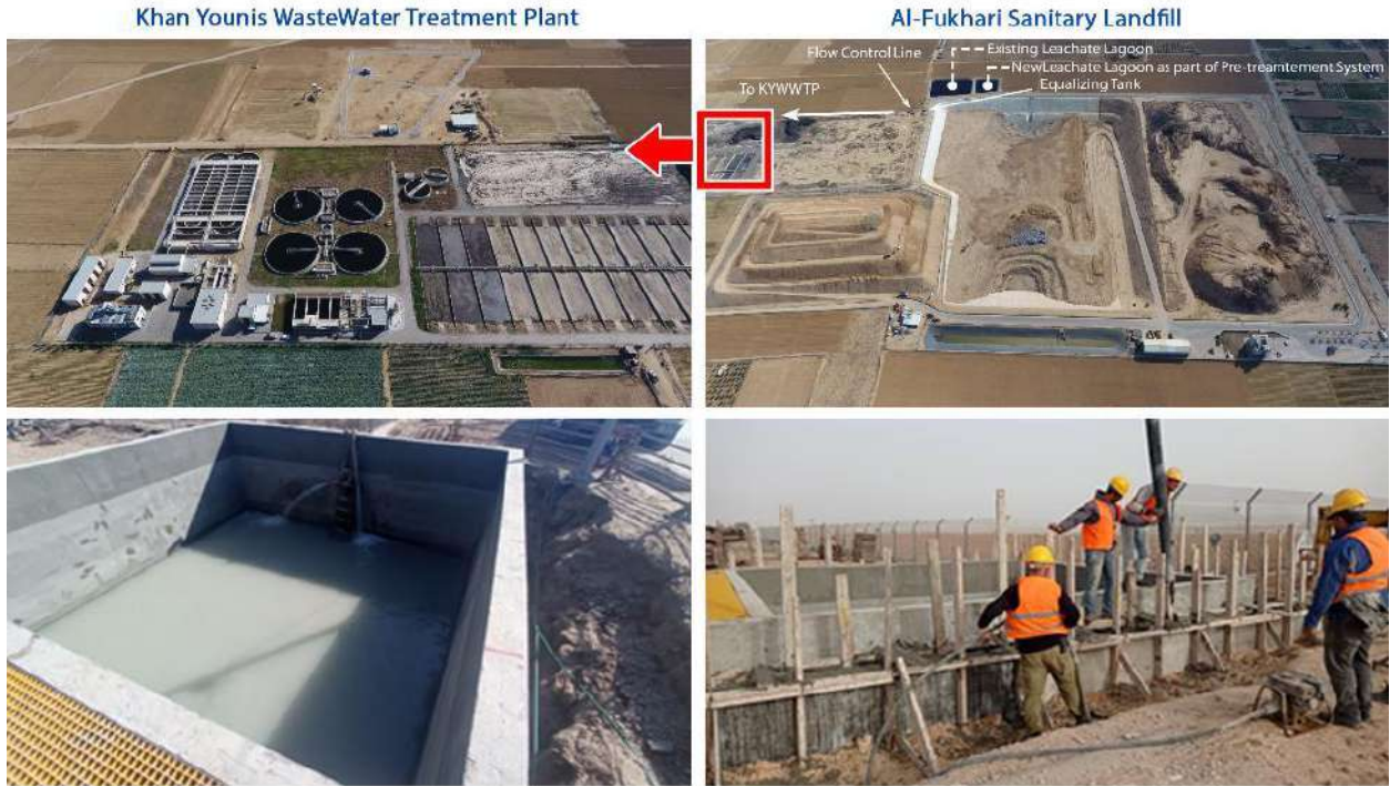
Leachate Pre-treatment System: June 2022 → (TOP) Landfill and WWTP, (BOTTOM) construction activities of leachate pre-treatment facility: equalizing tank, additional leachate lagoon, pressure lines & civil works
